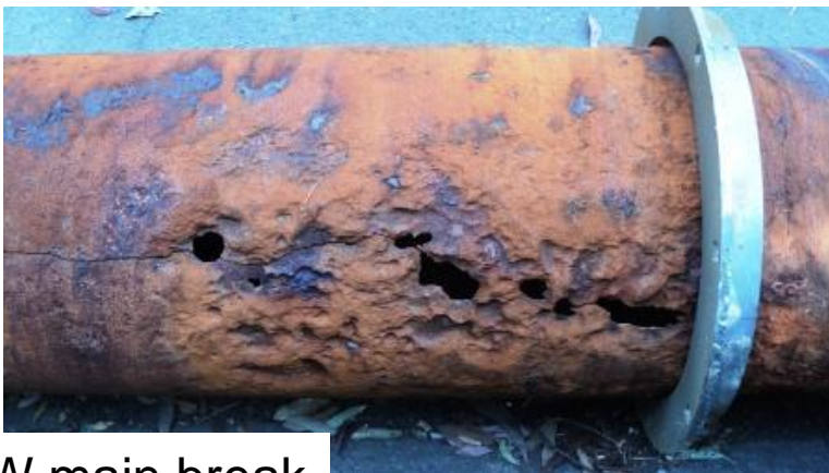
HW main break
