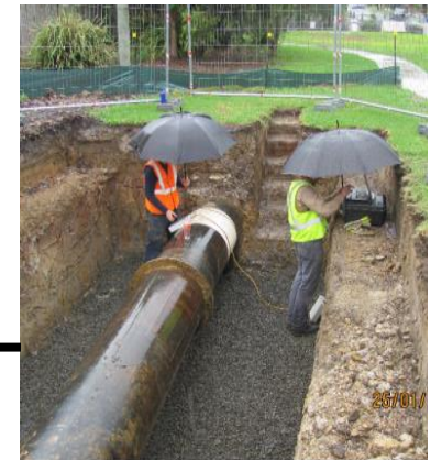
Testing data from pipe
