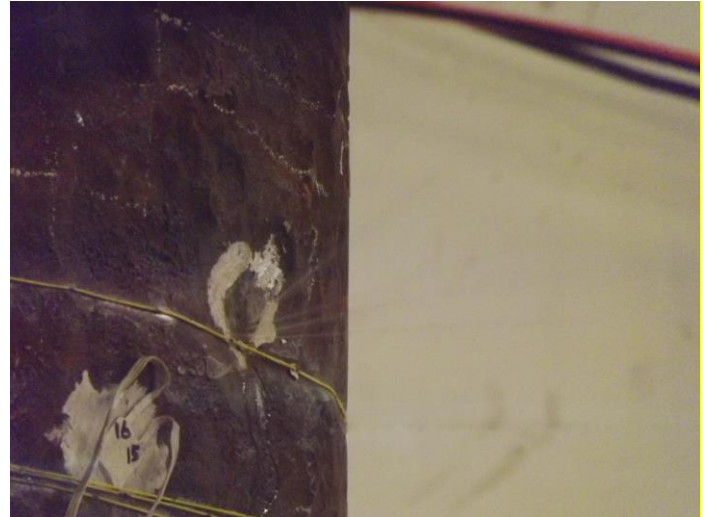
Figure 8. Water leaking from patch 3
