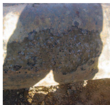
Figure 4 Patch corrosion (a) field observation and (b) visualisation of patch corrosion
