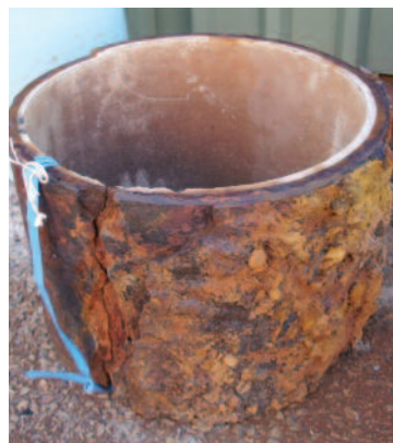
Figure 3 General corrosion: (a) field observation and (b) visualisation of general corrosion.
